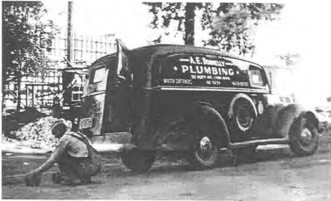
First sewer connection near Avalon Cafe, northeast of Golden Avenue and Lemon Grove Avenue, 1947. Photo courtesy of Lemon Grove Historical Society.
