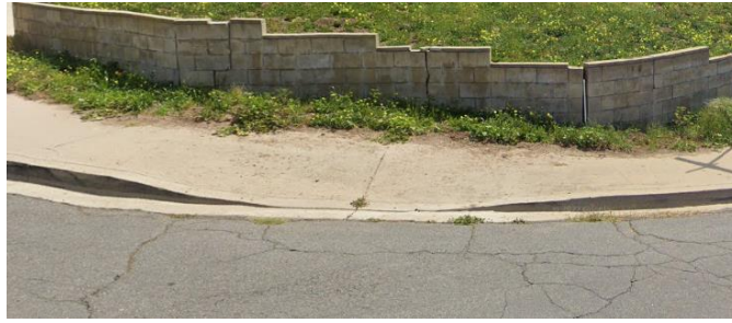
Not ADA Compliant
