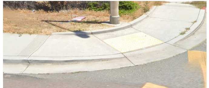
Meets Initial ADA Compliance
